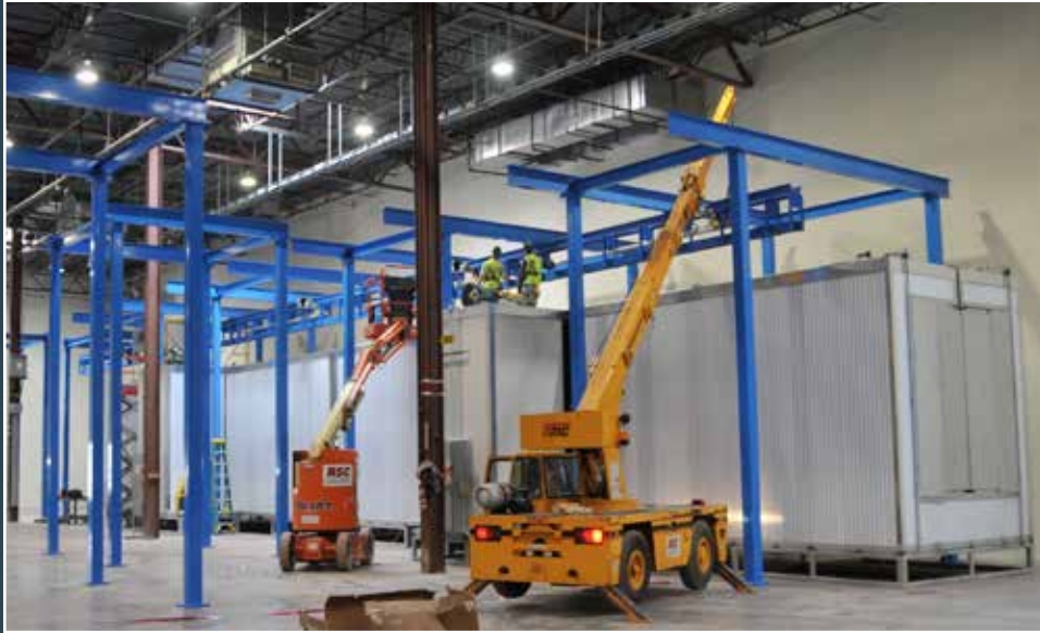
Modular construction allows for installation in half the time of conventional systems
